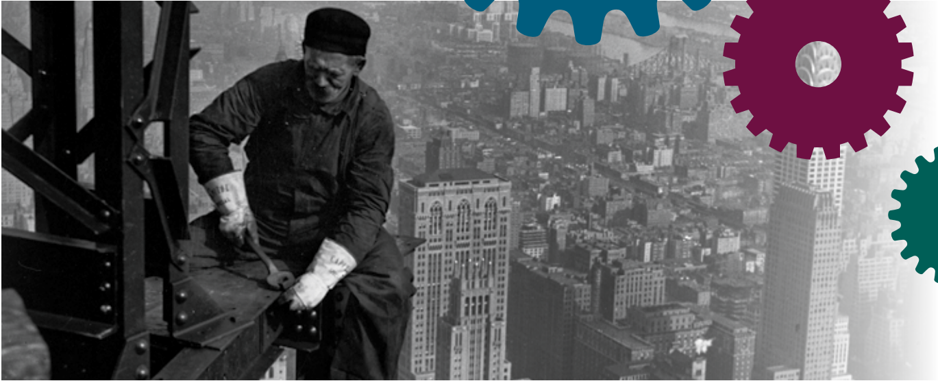
Workman on the framework of the Empire State Building, New York City, ca. 1930-31. National Archives, Records of the Works Progress Administration
